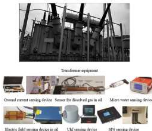
Fig.2 Various sensing devices for transformers
