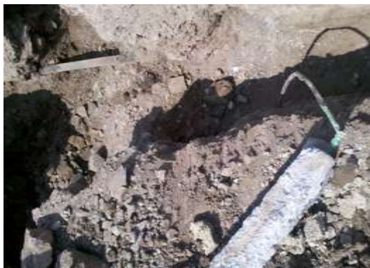
Fig 2: The sacrificial anode in the grounding grid.
