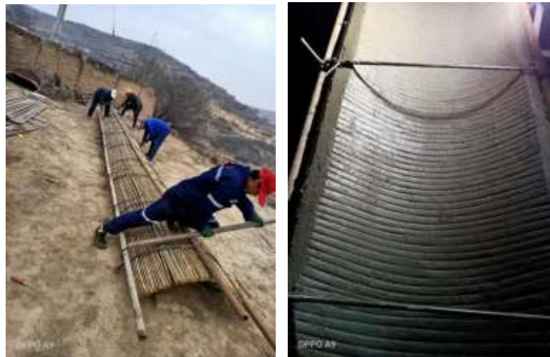
Fig 2: Formwork and inner wall scratch of concrete pipe.
