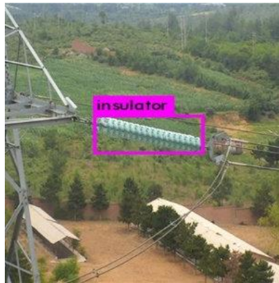
Fig.4 #319 Tower glass insulator self-exploding
