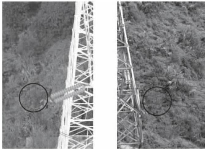
Fig. 5 Line wire anti-vibration hammer falls off
